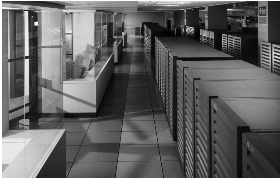
FIGURE 0-1 Simple, Clean, Modular Data Center Equipment Room
